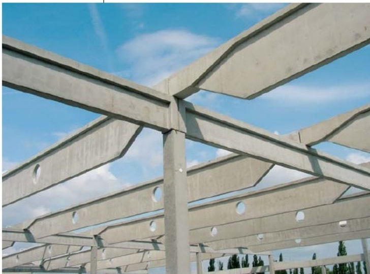
Fig. 6 Reinforcement of dapped end part of girder: (1) Main bars of looped at top, (2) Hairpins bars, (3) Support, (4) Elastomeric pad 300/130/10 mm
