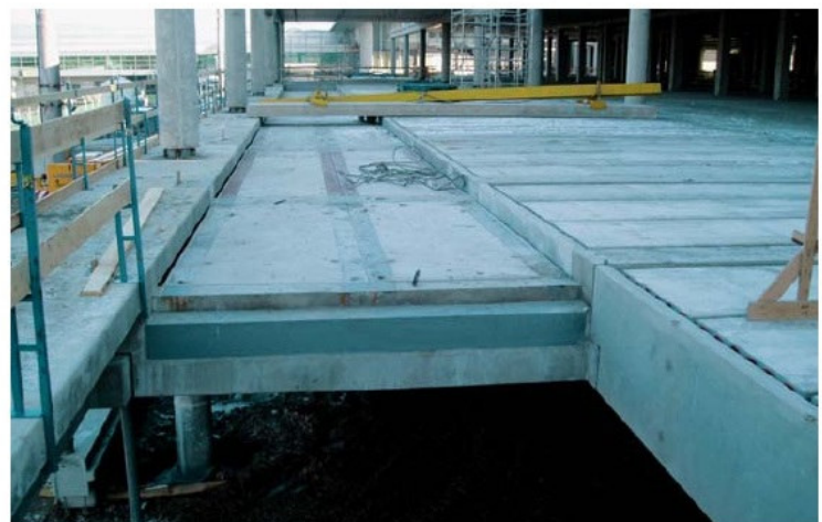
Fig. 3 View of a hollowing for travellers with an opening for the engine room Obr. 3 Pohled na vybraní pro travelátory s otvorem pro strojovnu
